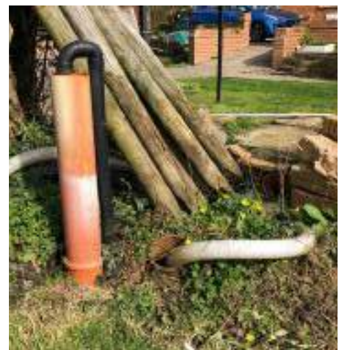
Rainwater runs through a series of French drains into a large sump into which a strong pump is fitted which pumps the water outside the garden boundaries.
