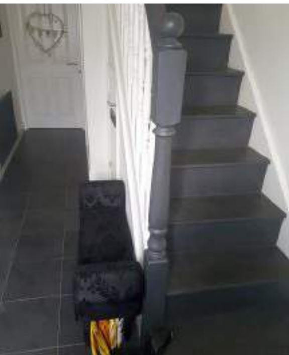
Tiling in the hall floor using waterproof adhesive and grout and removed stair carpet.
