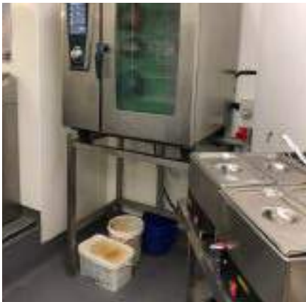
Vital kitchen equipment is raised above the flood water level.
