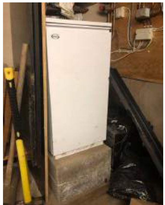
The boiler and freezer raised on a plinth.
