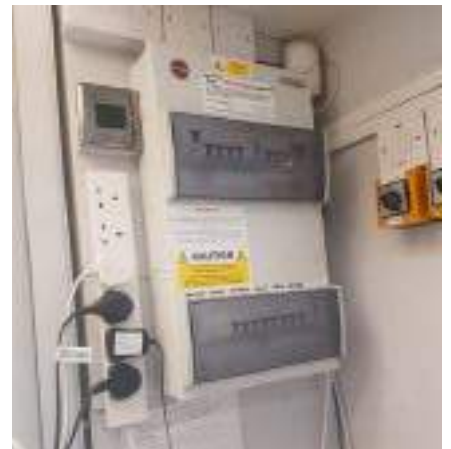
All electric service points are raised above flood level.
