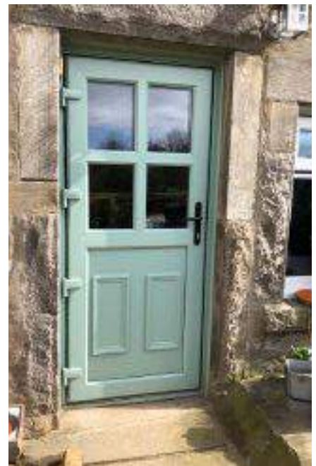
Flood door fitted.
