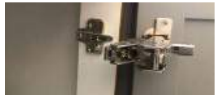
Kitchen doors have easy release hinges, so the doors can be removed quickly.
