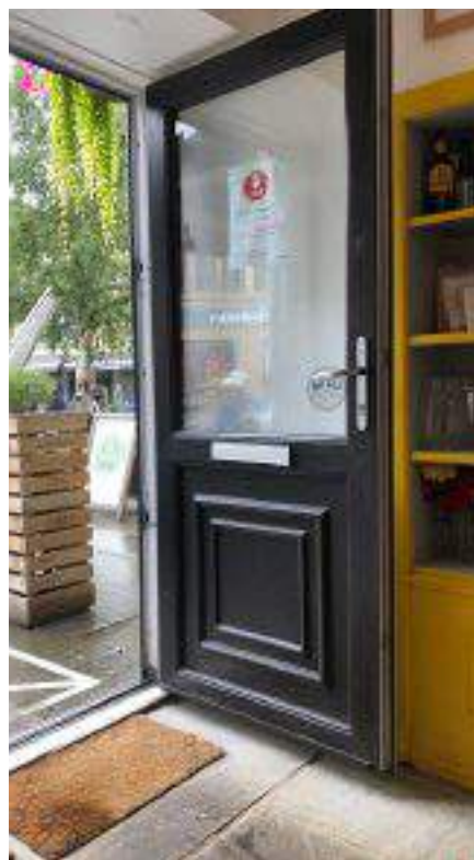
Kitemarked flood door and stone flagged floor.
