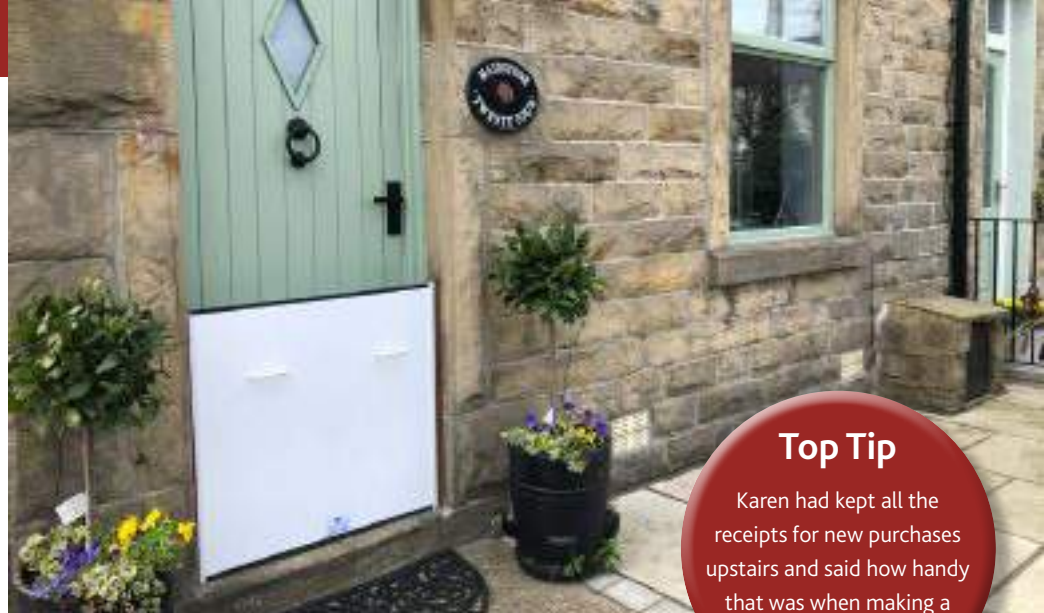
Flood Barrier to basement door and window.
