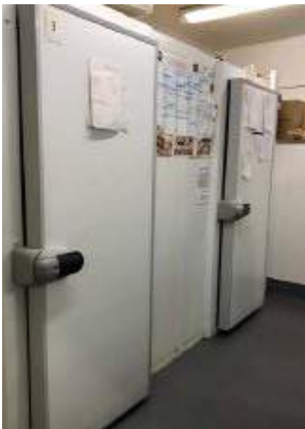
Cold stores have fitted rubber seals but in addition marine ply is sealed to the fronts.
