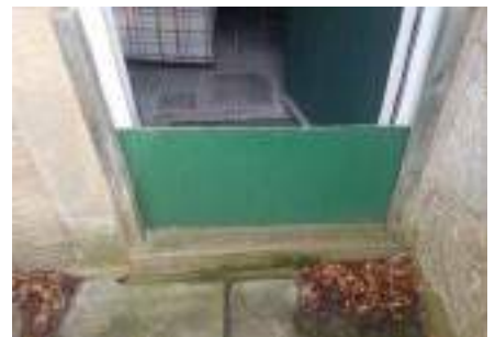
Home-made wooden ‘flood board’ which was effective in lesser floods.
