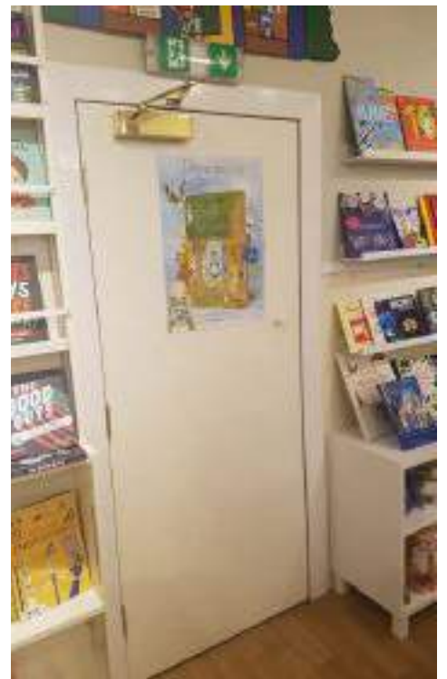
Plastic door architraves.
