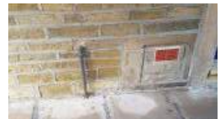
Walls were repointed and coated with a water proof spray and self-closing airbricks fitted.
