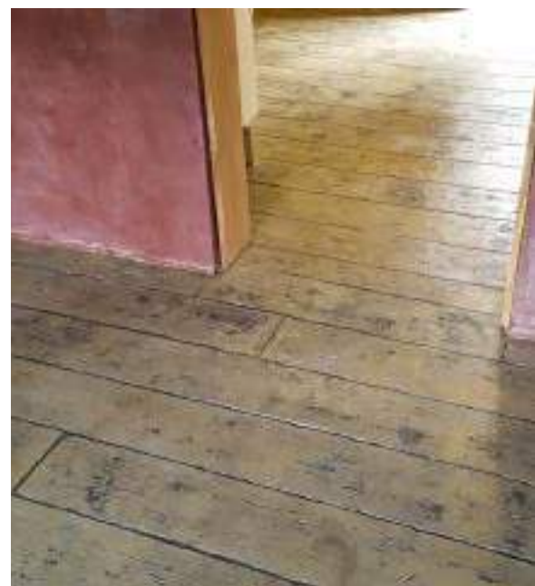
The floor is concrete, with an antique wood effect pattern, and sealed to give a gloss finish.
