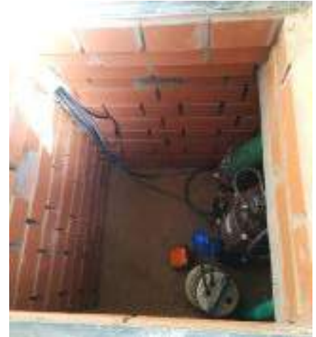
Two sump-pumps in lounge.
